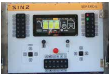
SINZ control panel.
